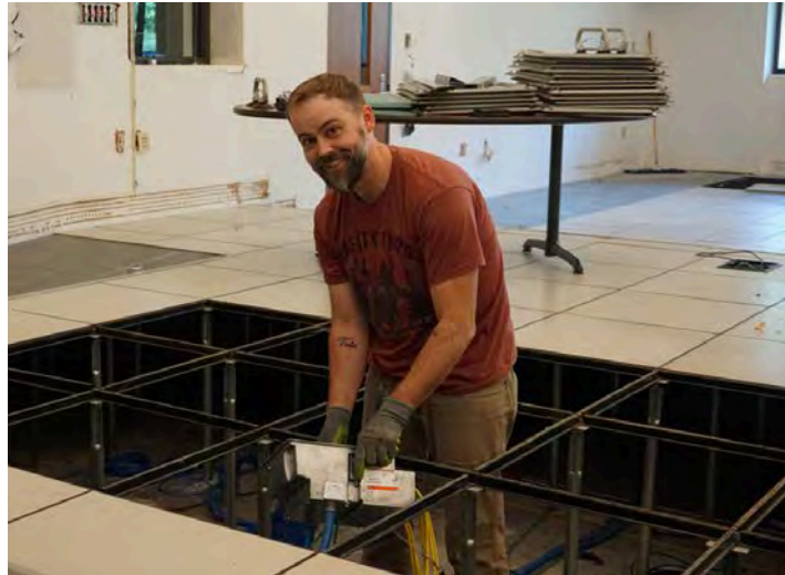
Kyle helping move wires in the dispatch floor
